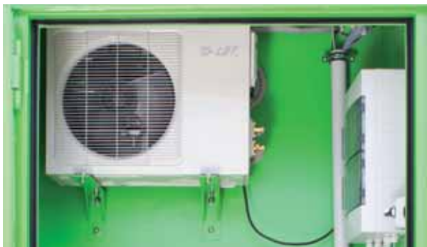
seperate functional niche with lockable door
